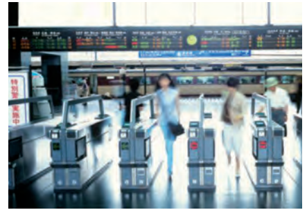
Access control and Ticketing
